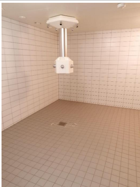
Duschen in Garderoben
