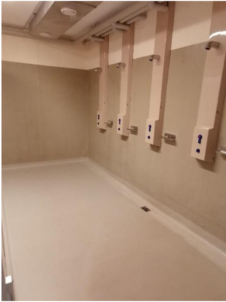
Duschen in Garderoben
