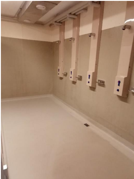
Duschen in Garderoben
