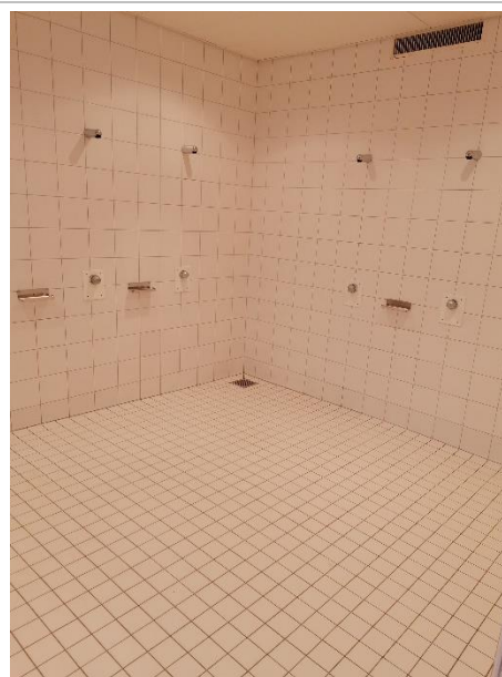
Duschen in Garderoben
