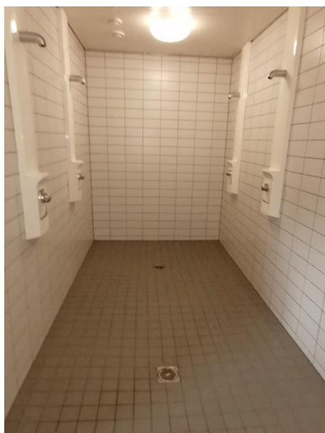
Duschen in Garderobe
