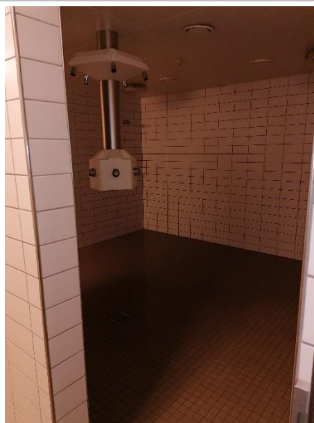
Duschen in Garderobe
